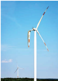
Example of a blade damaged by lightning.
